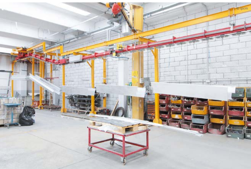
The monorail conveyor: this company coats iron, steel, galvanised steel, and aluminium components mainly for architecture.
