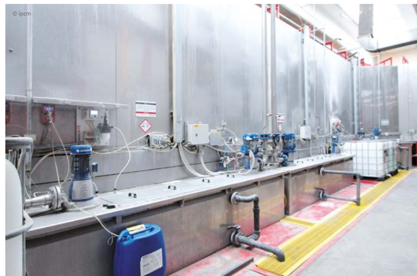
The pre-treatment tunnel
